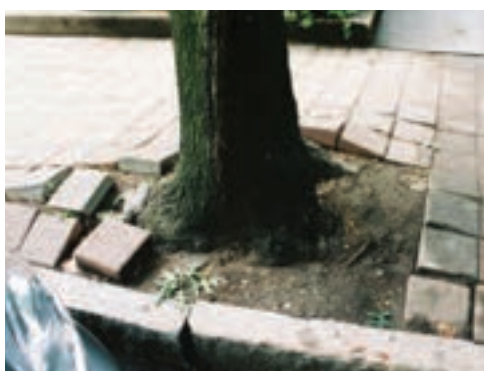
Before: Tree growth had buckled the surrounding bricks. Less than 5 feet between tree and building line. Frequent falls and lawsuits.
