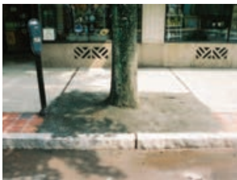
After: Poured concrete has replaced the bricks. Gravel around the trees allows for future growth.
